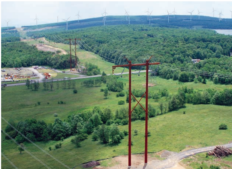
Two new steel H-frame transmission structures with a weathered finish stand between the pair of existing transmission lines. The NedPower wind farm, a joint venture of Dominion and Shell WindEnergy, Inc., is visible on the ridge.
